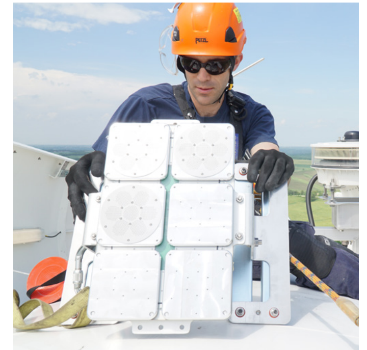
Technician installing an NRG bat deterrent system on the nacelle of a wind turbine. These ultrasonic emitters deter bats from the rotor-swept area keeping bats safe and optimizing energy production by allowing the wind farm to avoid curtailment.
