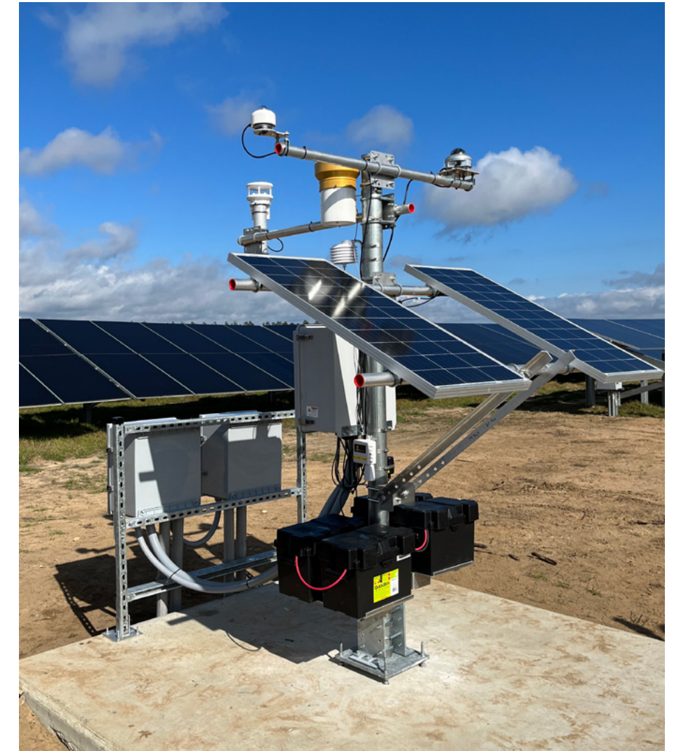
Solar Resource Monitoring (SRM) station installed at a solar farm for one of the largest solar developers in North America. SRM stations record similar measurements to SRA stations. The data is typically fed into the solar farm's local network as an input used to monitor and optimize the ongoing performance of the solar farm.
