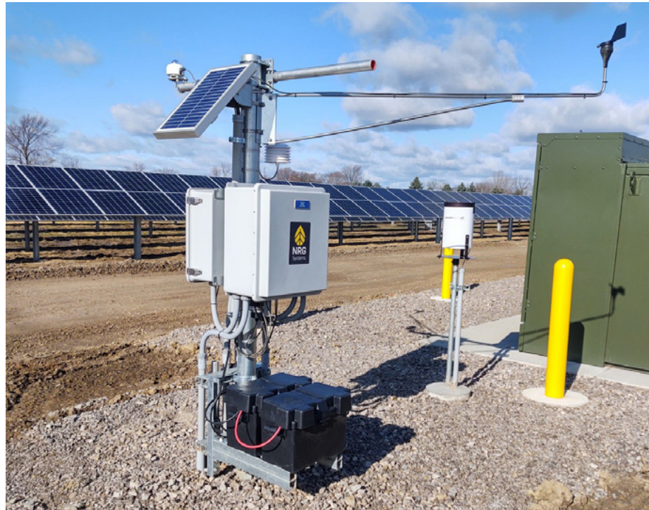
Image of an NRG Solar Resource Monitoring System on a Solar Farm. NRG offers various Flare SRM Station configurations to suit customers' site-specific needs.
