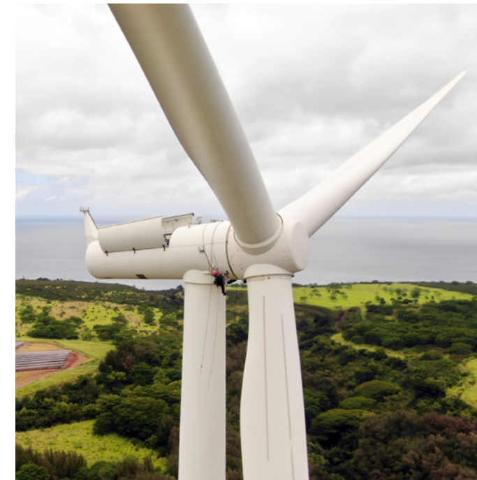
Technicians installing an NRG Bat Deterrent System at the Kawaihoa wind Farm in Hawaii. Each turbine will have deterrent units pointing in several directions to ensure coverage of the entire rotor-swept area.
